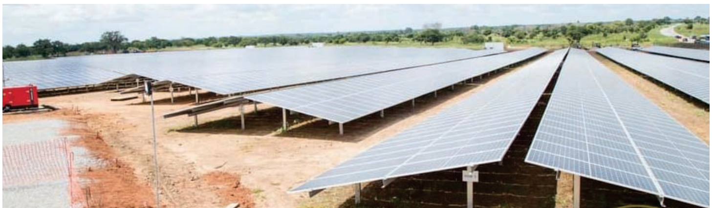
The Lawra Solar Panels
